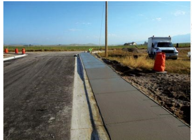
The Confederated Salish & Kootenai Tribes constructed this road improvement project to access home sites on the Flathead Reservation.
