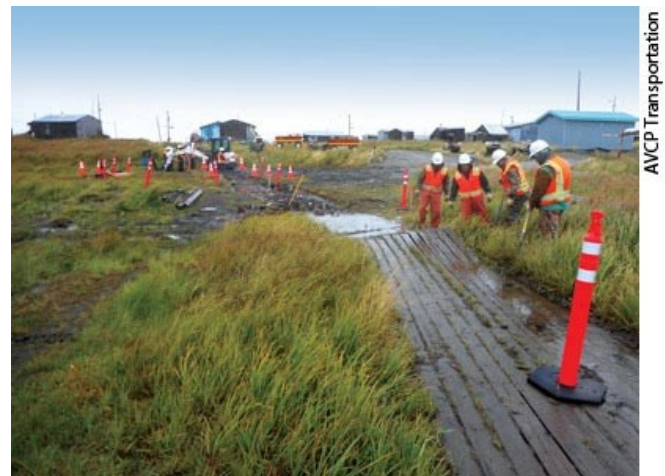
These workers with the Association of Village Council Presidents are constructing an old boardwalk at Kongiganak, a coastal Alaskan village.
