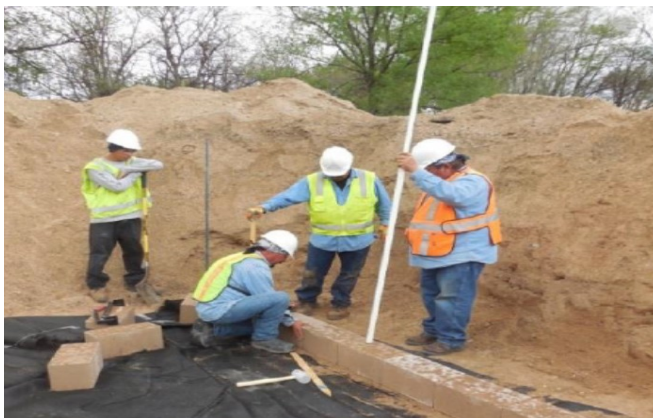
An Ohkay Owingeh road crew used GRS-IBS to replace the White Swan Bridge
